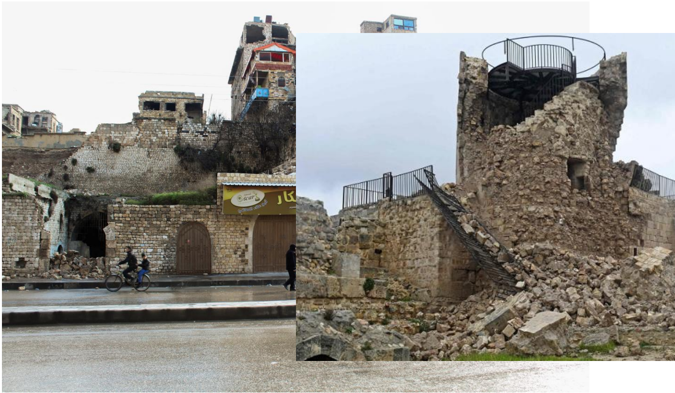
Figure 5. Images of earthquake impact on Aleppo Old Citadel (left) and Al-Marqab castle (centre) in Syria.
