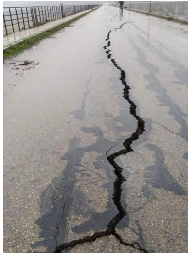
Figure 11: Image of the cracks on the Maydanki (Afrin) Dam (source: @hybacarm)
