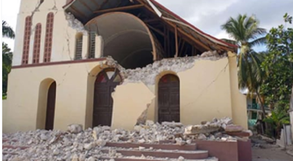
Fig. 13 - Damage due to the earthquake (source: private communication).
