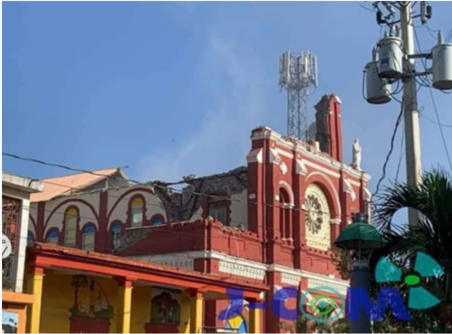
Fig. 11 - Damage to the Cathedral in Jeremie (source: J-COM news site).
